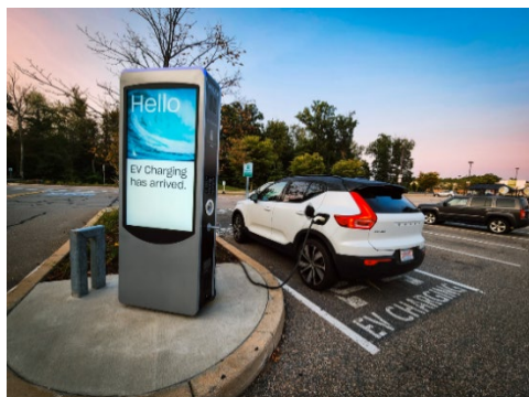
PICTURE 5A-2. EV CHARGING STATION
