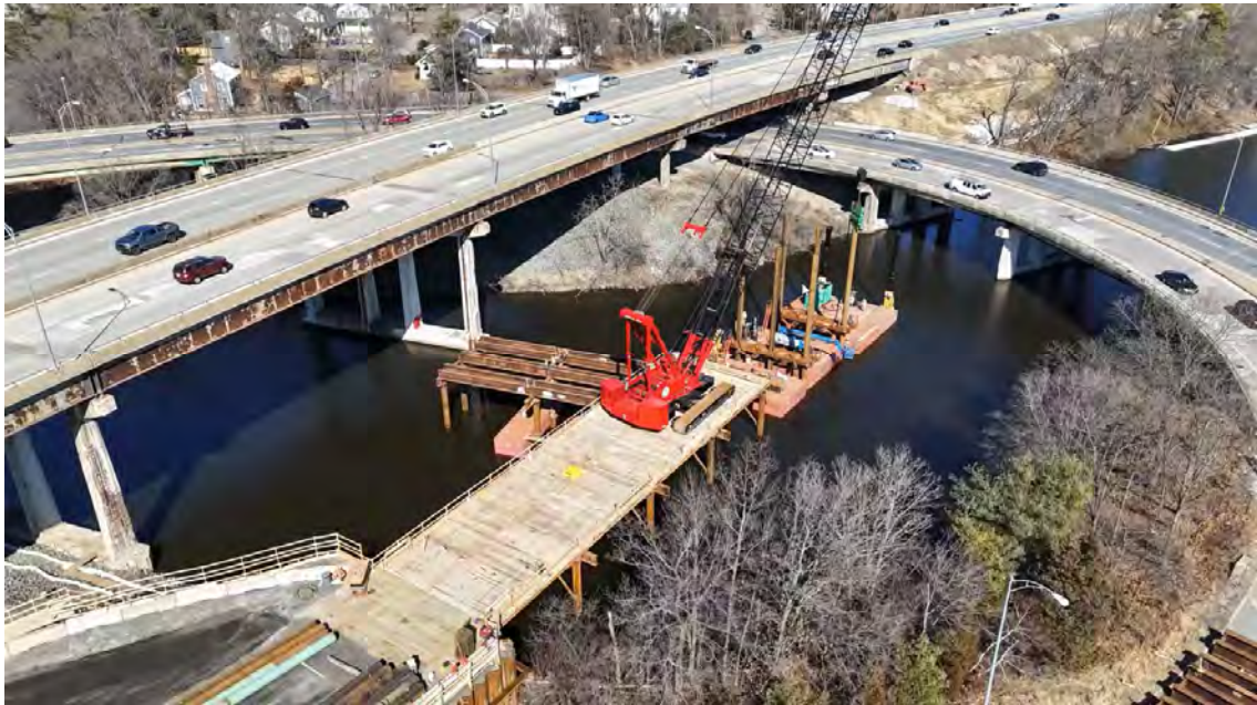
Begin Construction of South Bulkhead and Trestle Providing Access across Charles River
