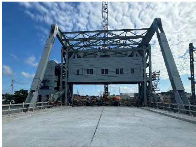
Moveable span, link arms, Machine Room August 2024
