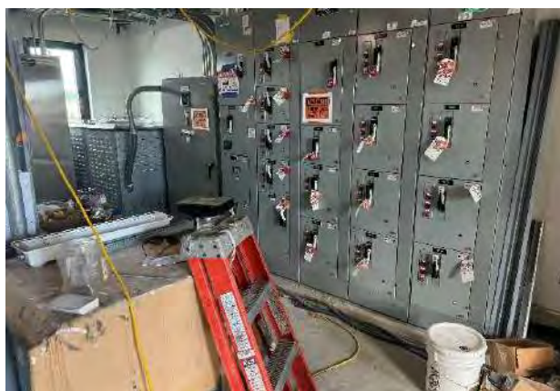
Control House August 2024
