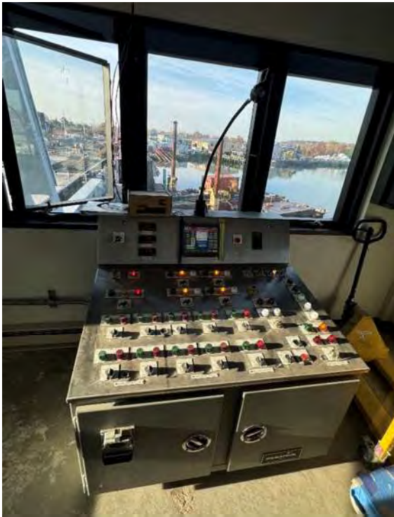
Control House October 2024
