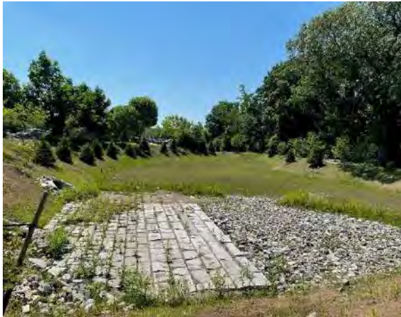
BMP 30 at the entrance to 770 Dedham Street June 2024
