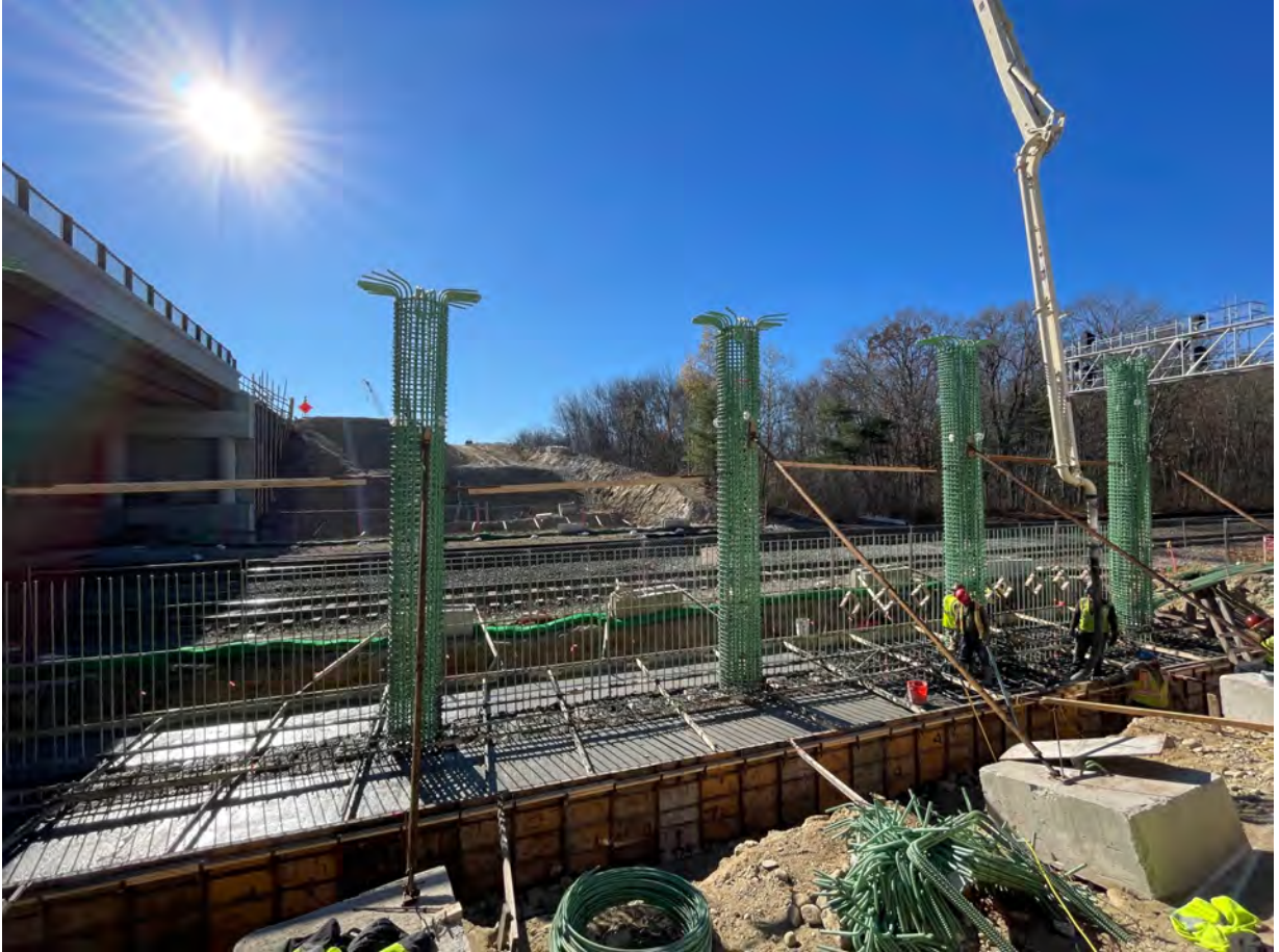
495 Southbound over RR with temp 495S on new bridge in median (left)
