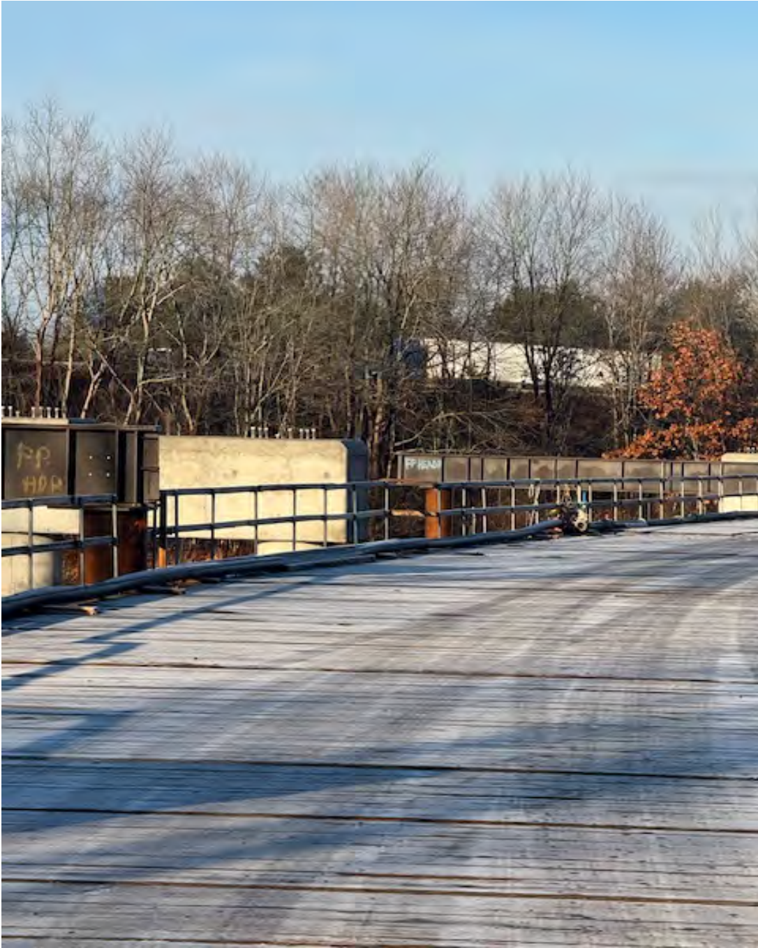
Ramp WN concrete piers and falsework ready for bearings and tub girders
