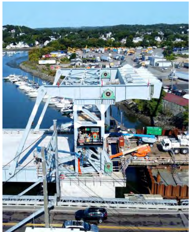
Tower, counterweight girder, link arm, Machine Room September 2024
