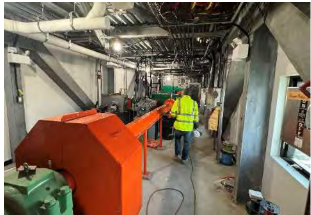
Machine Room interior October 2024
