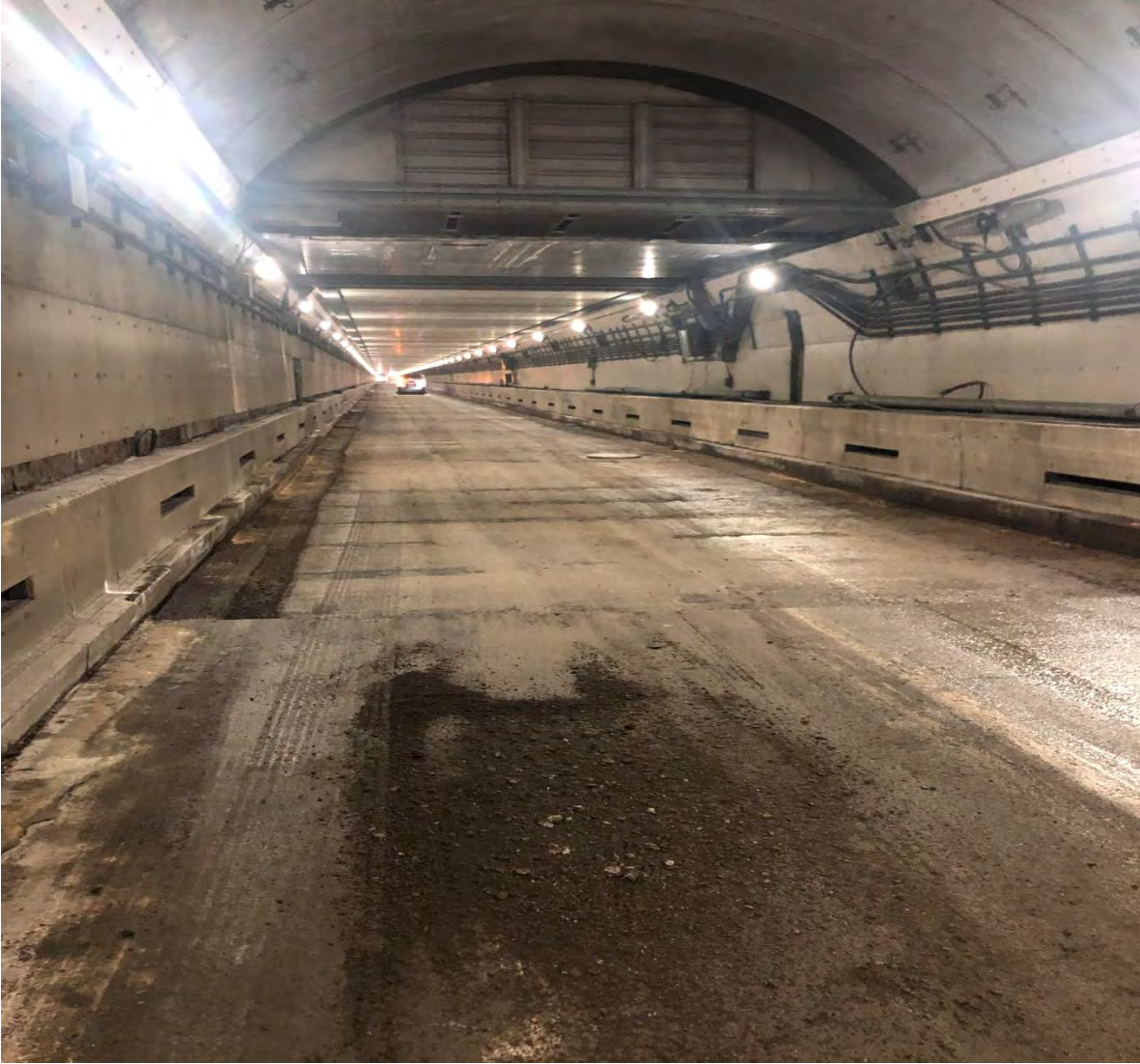
PHOTO THREE (below): photo of tunnel just before final paving was installed
