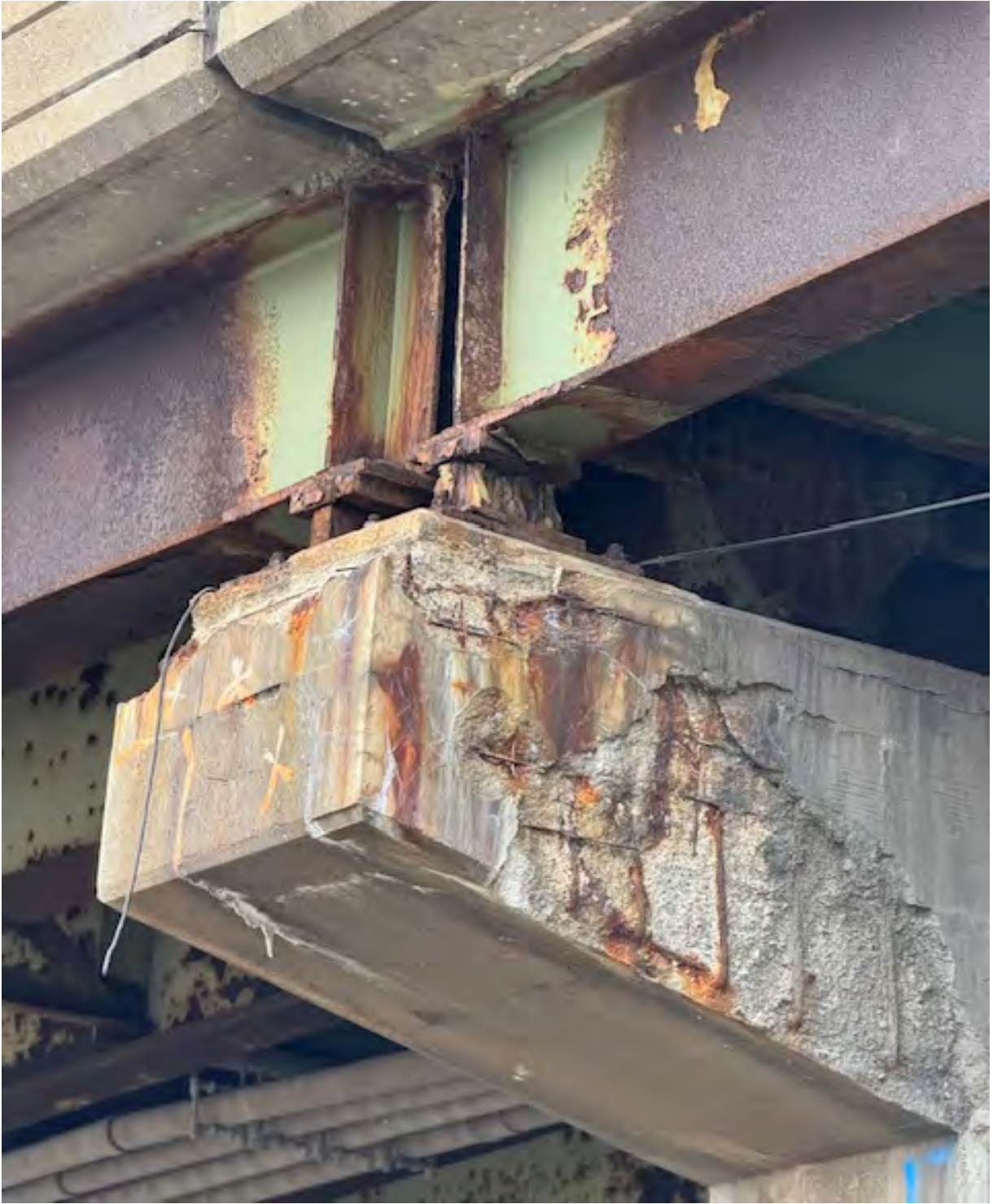
Typical conditions of concrete pier cap and steel beams prior to repairs (2023)
