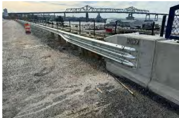
F-02-087 SW endpost and guardrail October 2024
