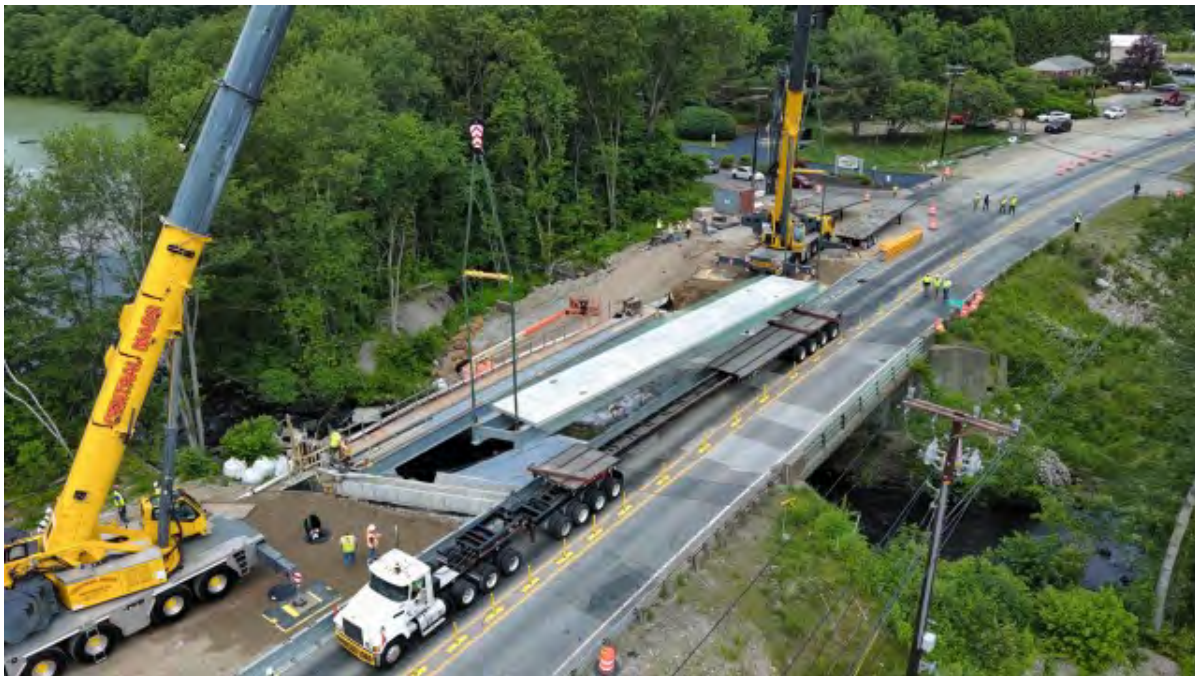
Precast Bridge Units Installation with Rolling Road Block - French River Bridge Stage 1
