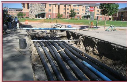
8" dia. Pipes between Central Loop And H.H
